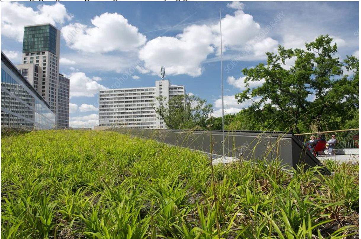
Figure 4 Green roof, Berlin, Germany (library, 2024)
